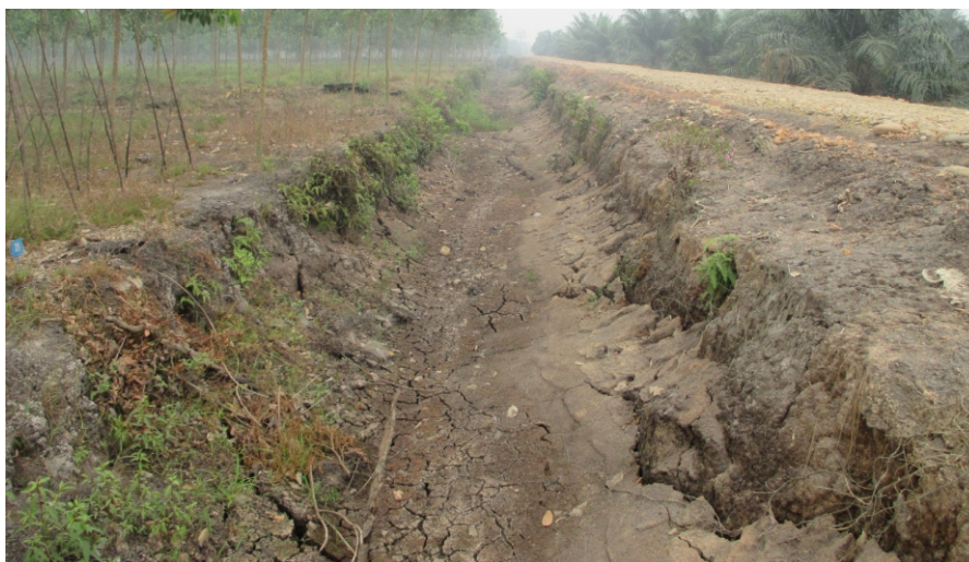
Gambar 2. Kondisi saluran drainase Oktober 2015 Figure 2. Condition of the drainage channel in October 2015
